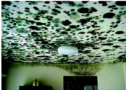
Photo 2: Extensive mold contamination of ceiling and walls
